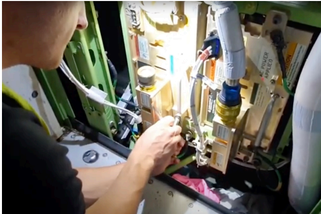
Supplementary cooling unit
