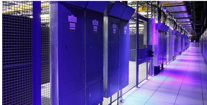
Data centers are neutral places housing equipment from multiple (cloud) providers in separate 'cages'
